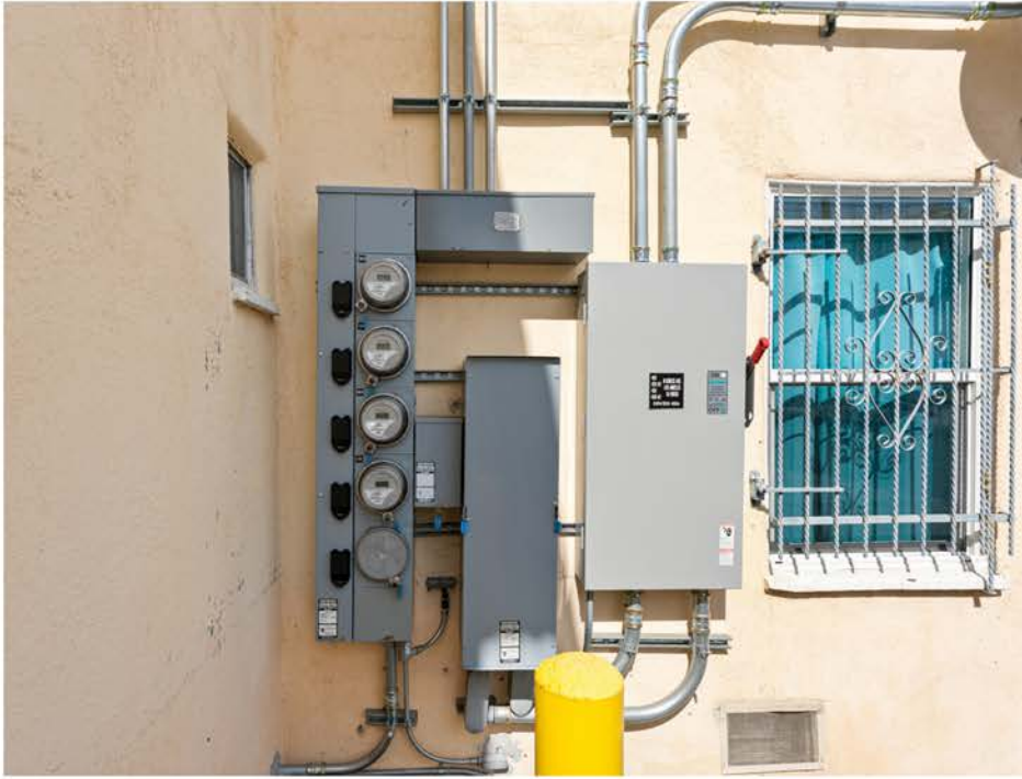
Recently Upgraded Electrical Panels
