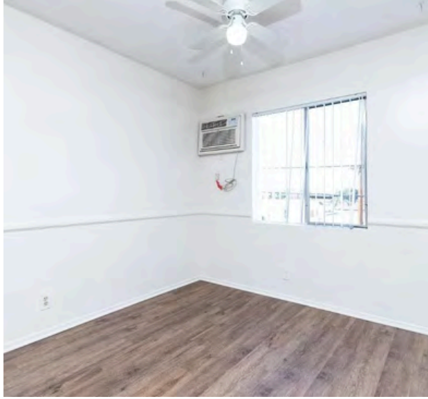
Wall AC and Window
