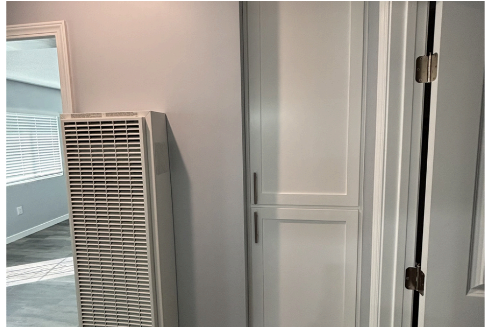
Wall Heater and Storage Space
