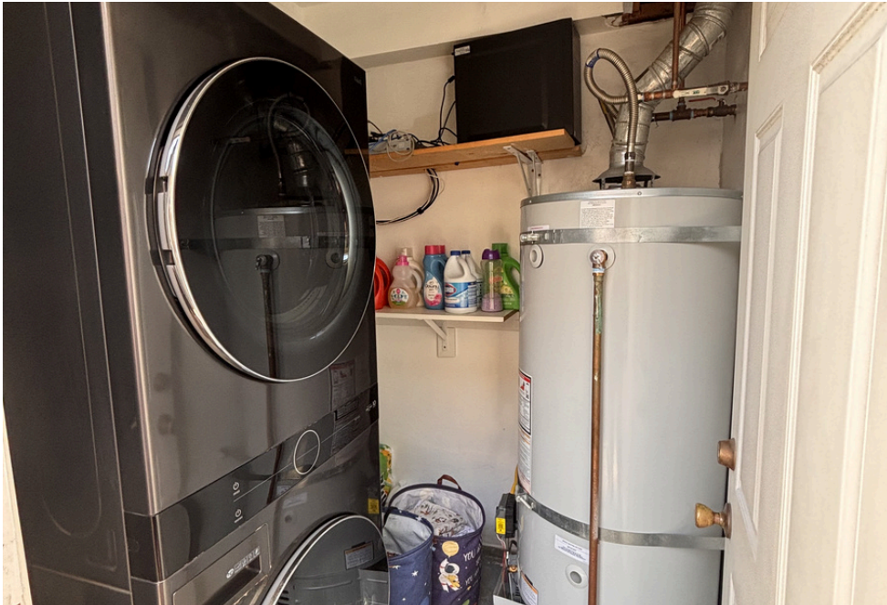
Laundry Room and Water Heater
